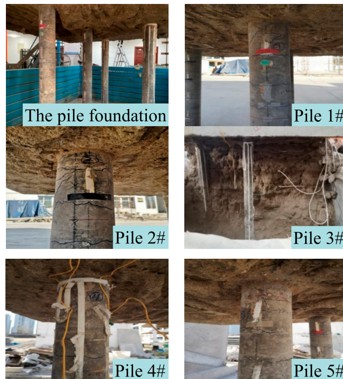
Figure 8. Status of piles in hard soil site after the test.
