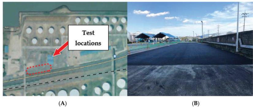
Figure 6. (A) Location of test construction in GS Caltex Complex, Yeosu city, South Korea and (B) View of test construction.
