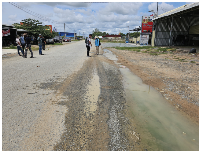
Figure 12. Deterioration on the edge of the testbed.
