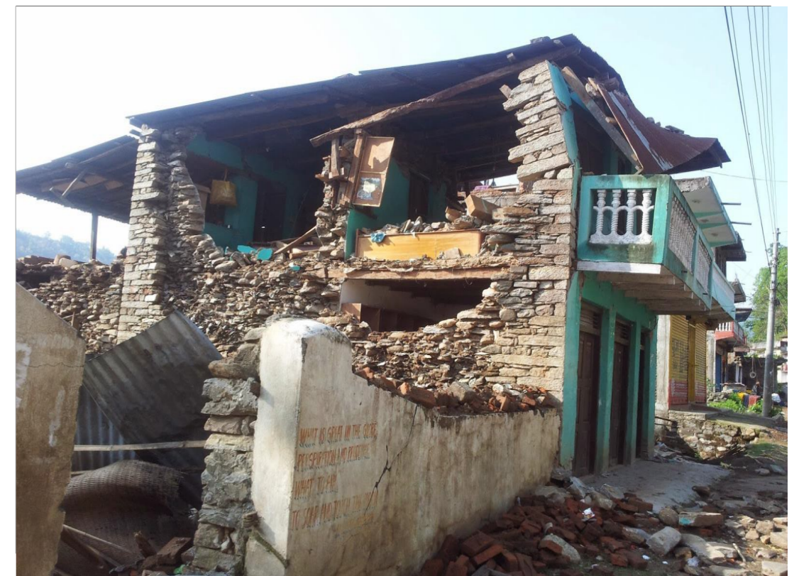
Figure 1. A house damaged by the earthquake in Gorkha district, Nepal.
