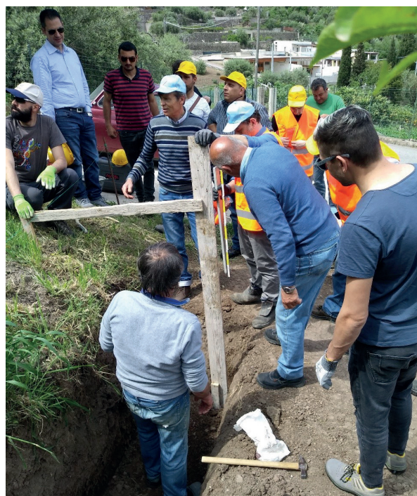
Figure 3. Master builders showing how to prepare guides for regulating the slope of the wall before its construction (Photo by A. Sardella)
