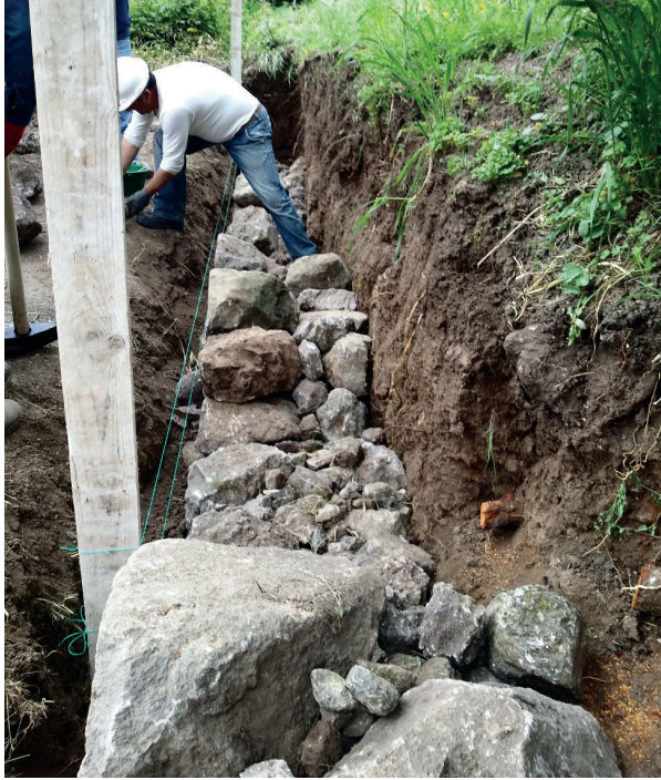
Figure 4. Practitioners positioning the drainage internal filling of the wall with smaller stones. (Photo by A. Sardella)
