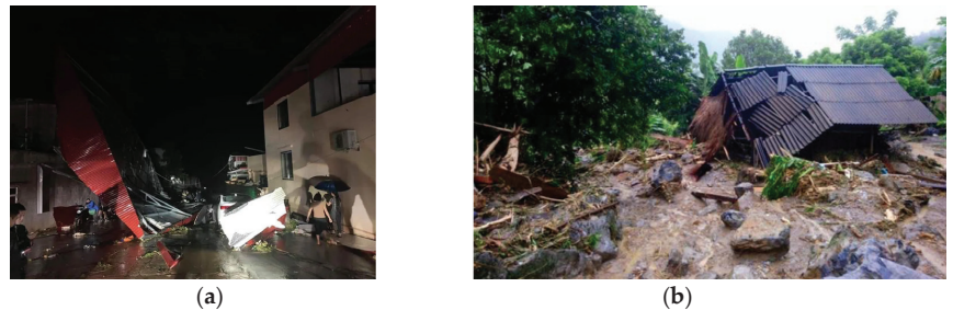
Figure 2. This is the damage to buildings in urban (a) mountainous settlements (b) caused by heavy rainfall and strong winds in Yen Bai Province in 2023.
