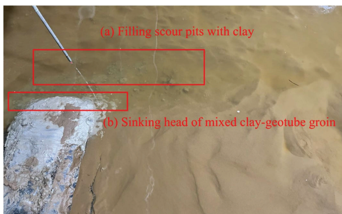
Figure 20. Scour pit at the head of the mixed clay–geotube groin.
