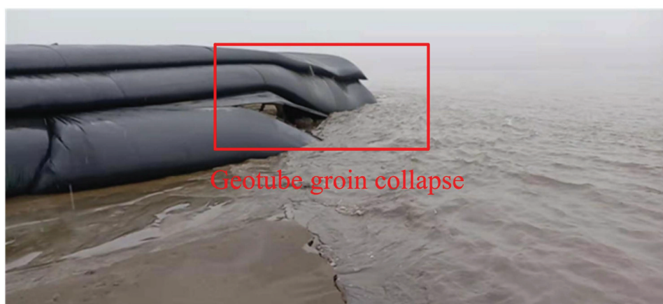
Figure 2. Geotube groin collapse.
