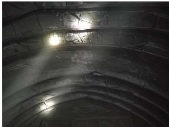
Figure 11. The twisted steel arch and back haunch fillet of the arch, and rockfall of the initial support.
