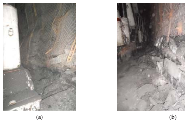
Figure 6. Spalling failure of protective coal pillar in the main recovery room: (a) panel 15205; (b) panel 15206.
