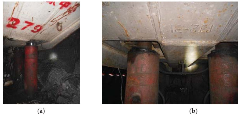
Figure 1. Large deformation of roof and hydraulic support crushing accident of a recovery room in Shennan mining area: (a) less than 100 mm stroke of hydraulic support column; and (b) completely crushed hydraulic support.
