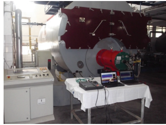
Figure 1. Boiler under measurement and test set-up.
