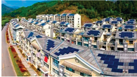
Figure 12. Rooftop photovoltaic installation in Li’ao Village.
