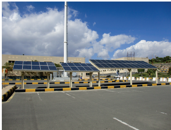
Figure 2. The Installed solar PV system at KKU.
