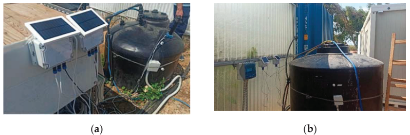
Figure 16. Monitoring of water quality: (a) seawater tank; (b) irrigation tank.
