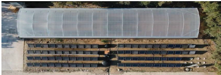
Figure 15. Solar power desalination system.
