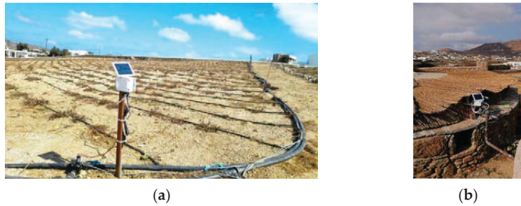
Figure 10. (a) Electrovalve for controlling the water flow; (b) Level sensor installed in one of the tanks.
