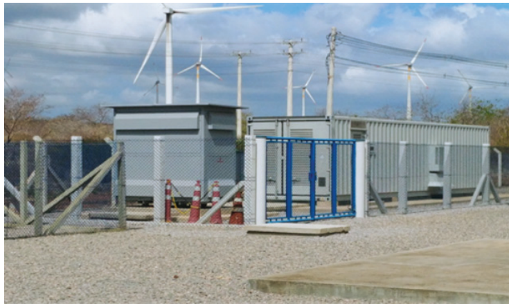
Figure 2. Installation of BESS in the Campo dos Ventos Substation.
