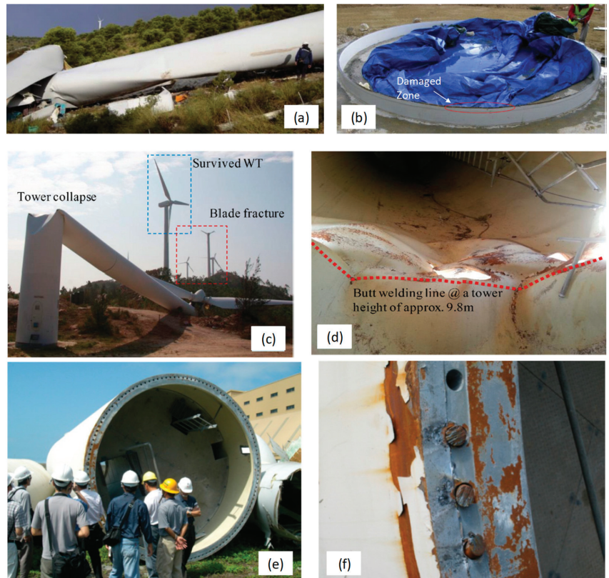
Figure 4. (a) The scene of the wind turbine tower collapsed at the wind farm Abuela de Santa Ana, Spain caused by joint failure. (b) The view of the damaged joint where the failure began. (c) The structural failure of a wind turbine tower in China's Shanwei city caused by super typhoon Usagi. (d) The view of local buckling of the tower at wall-thickness transition zone. (e) The view of the fractured tubular tower section of a wind turbine in Taiwan. (f) The scene of fractured bolts ((a,b) adapted from [65], (c,d) adapted from [67], and (e,f) adapted from [4]).
