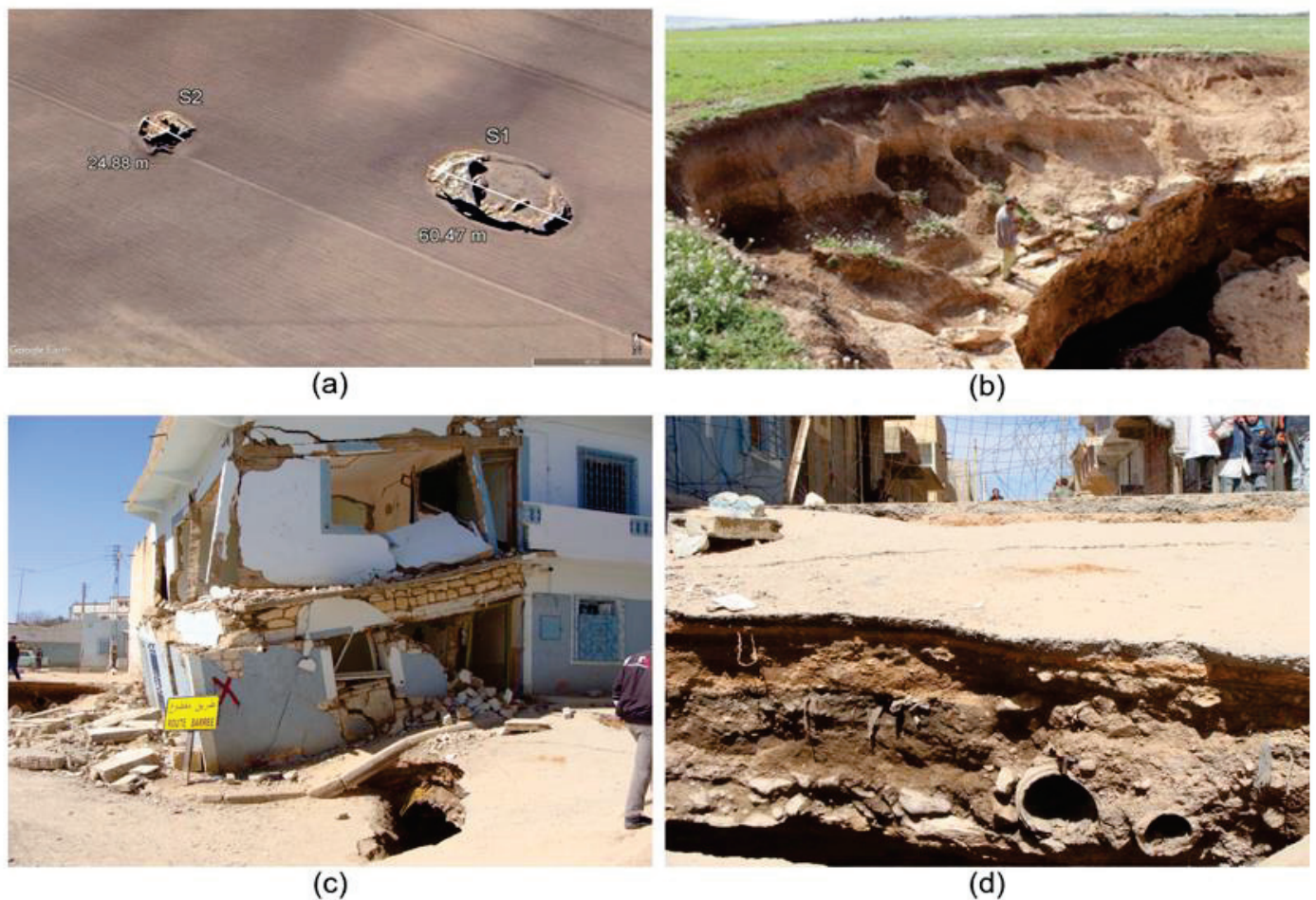
Figure 3. Sinkhole example images: (a) Draa-Douamis sinkholes 1 and 2 collapsed with a diameter of 66.47 and 24.88 m, respectively (location: see Figure 1—sinkhole sites; date: during 2004); (b) example of sinkhole diameter enlargement in surface; (c) Harkat Bouziane sinkhole collapsed in the city with a diameter of ~50 m and height of 2 m (location: see Figure 1—sinkhole sites; date: February 2009), destroying infrastructure; and (d) damage created by a sinkhole event (i.e., sewer network and roads broken).
