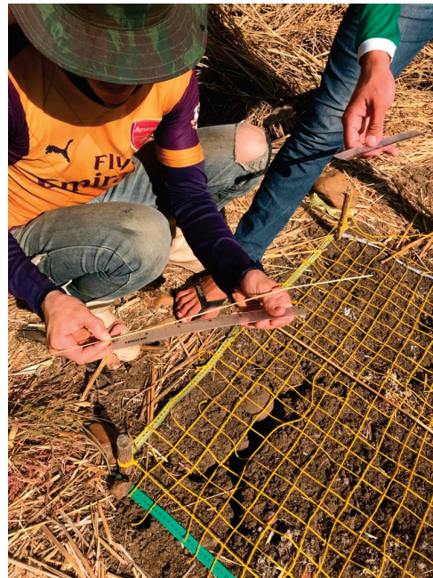
Figure 4. Crack monitoring in situ.
