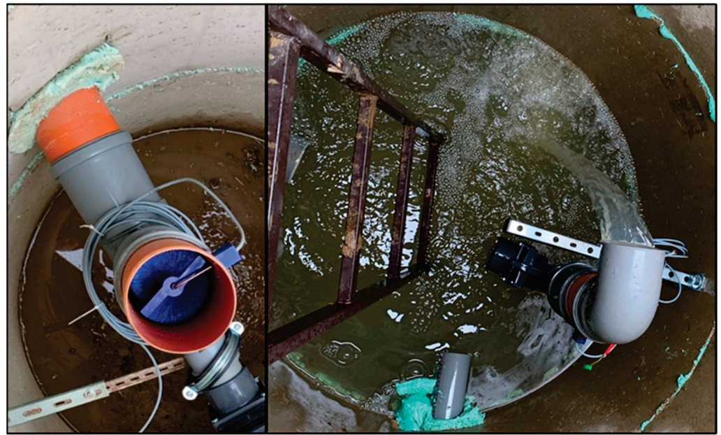
Figure 3. Fixed WLCS installed in the manhole with propeller flow meter (left) and water overflow after a rainfall-runoff event on 14 May 2021.
