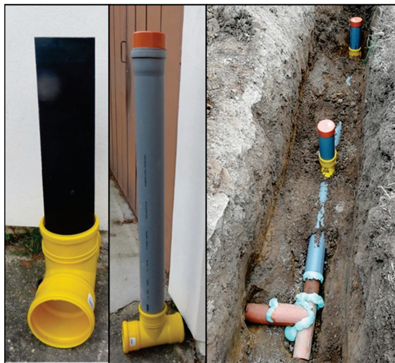
Figure 2. Underground fixed WLCS consisting of a drainage T branch (yellow), a polypropylene gate (black) and a PVC pipe vertically connected to the T branch (grey) with a cap (brick-red); before and after installation on tile drainage.
