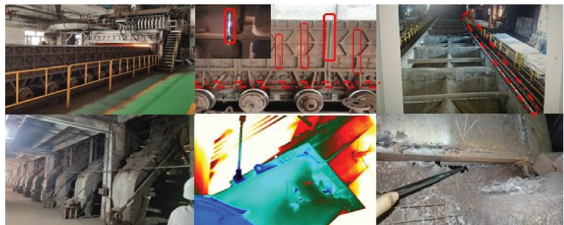
Figure 2. Some typical leakage in region A.
