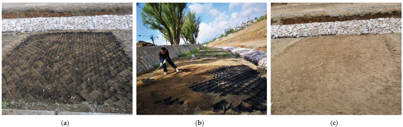
Figure 8. Infilling of the top soil: (a) bottom 10 cm of bare soil; (b) infilling from the crest to the toe; (c) the finished slope after treatment.
