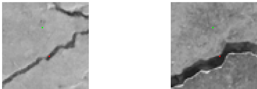
Figure 13. Samples covered by a rule of class ‘Cracks’; rule antecedents are represented by colored dots. The top left shows the centroid of the 4549 covered samples in the training set. The other pictures show three of the one thousand one hundred twenty samples in the test set that activate this rule.
