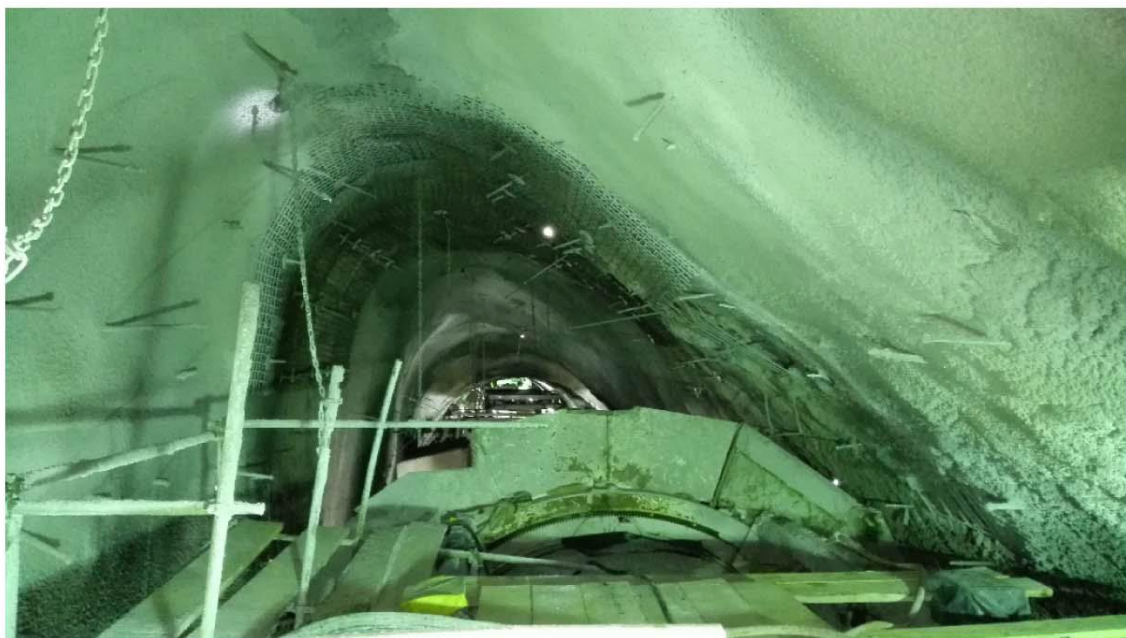
Figure 8. Over-excavation profile of the headrace tunnel after the rock burst on 31 May.
