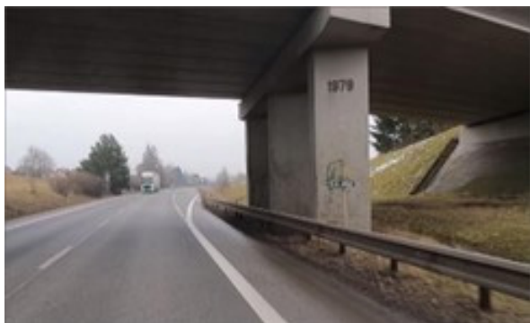
Figure 3. Insufficient minimum distance behind the crash barrier.
