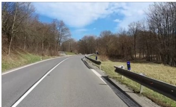
Figure 2. Incorrect beginning/end of the crash barrier.
