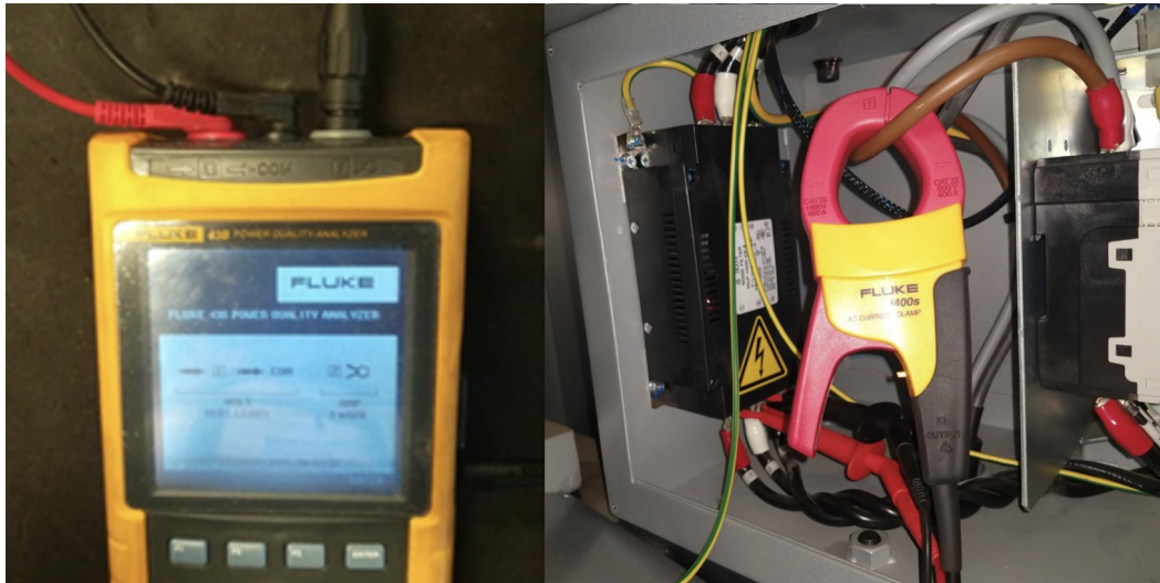
Figure 4. Connection of the power analyzer (Fluke 43B) on the main lines of the Zodick VZ300L machine.
