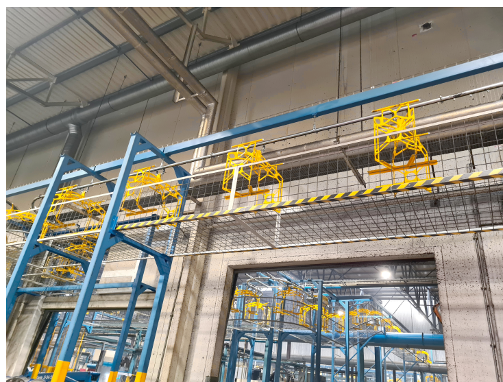
Figure 27. Overhead conveyor with new carrier.
