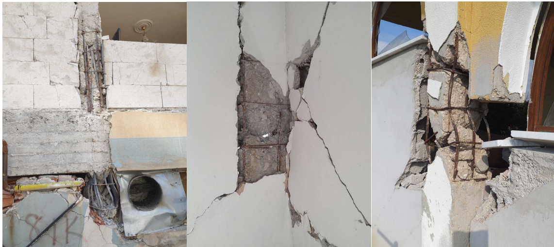
Figure 3. Examples of damage caused by insufficient concrete cover.
