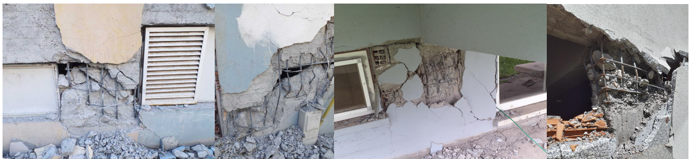
Figure 2. Examples of damage by low-strength concrete.
