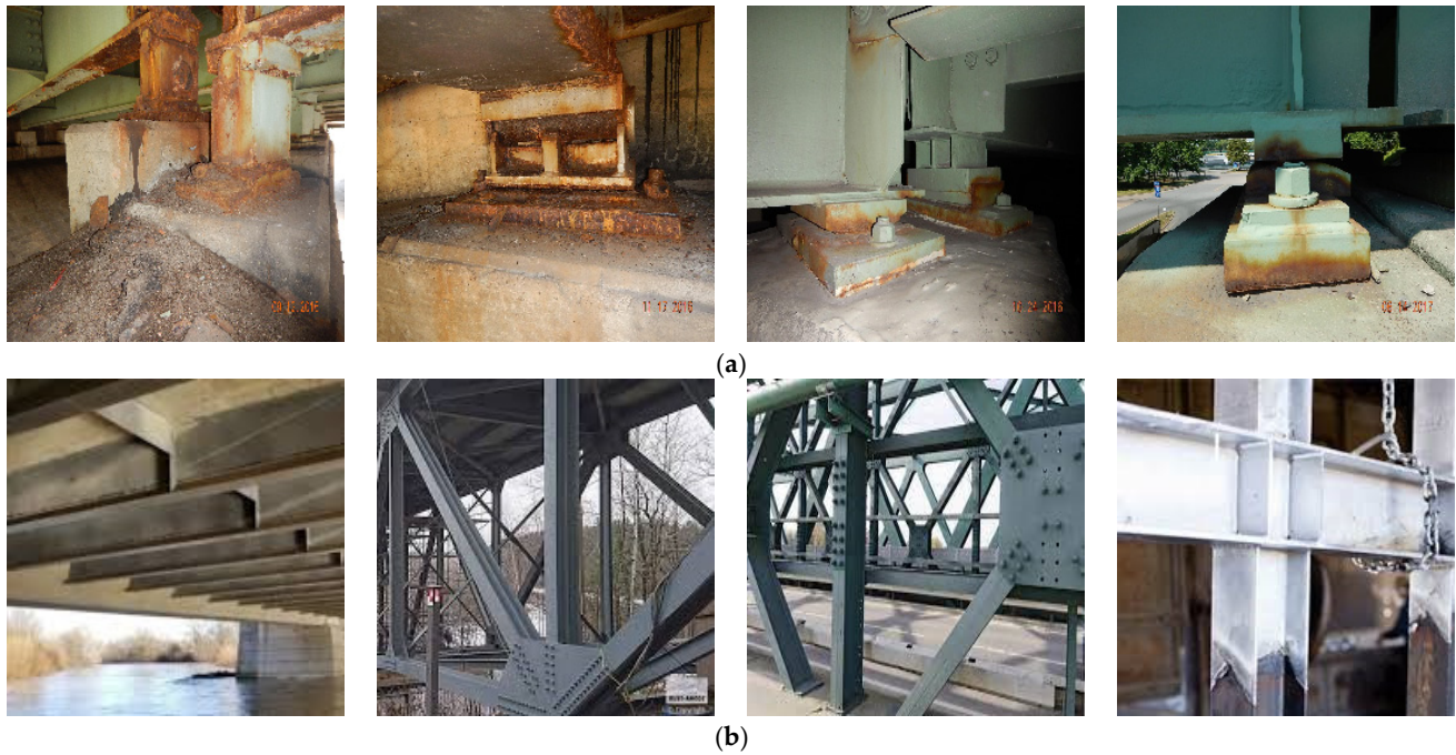
Figure 12. Dataset examples of the (a) corrosion and (b) no-corrosion classes.
