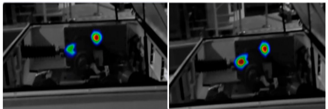
Figure 12. AIS partial discharge of EMU under AC withstand voltage.
