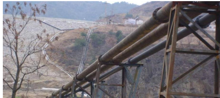
Figure 6. High-head double-line tailings conveying project of a mineral processing plant.
