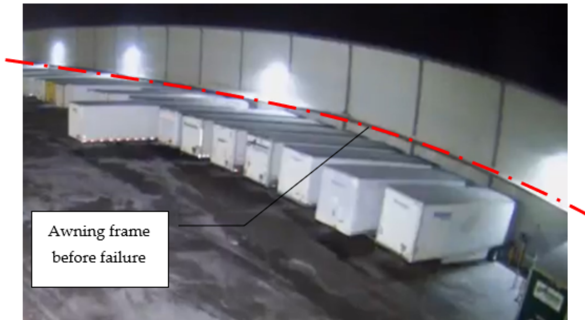
(a) Awning frame before failure
