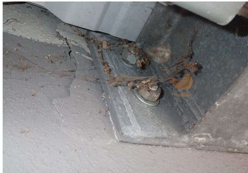
Figure 4. Insufficient length of embedment.
