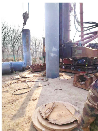
Figure 6. Depth markers on the pile sides.
