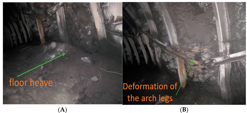
Figure 10. Results of field visual observations in the ventilation drift 334D6-1-v of the Kazakhstanskaya mine: (A) floor heave concentrated on the right side; (B) deformation of arch support legs, extrusion of sidewall rocks, and failure of struts.
