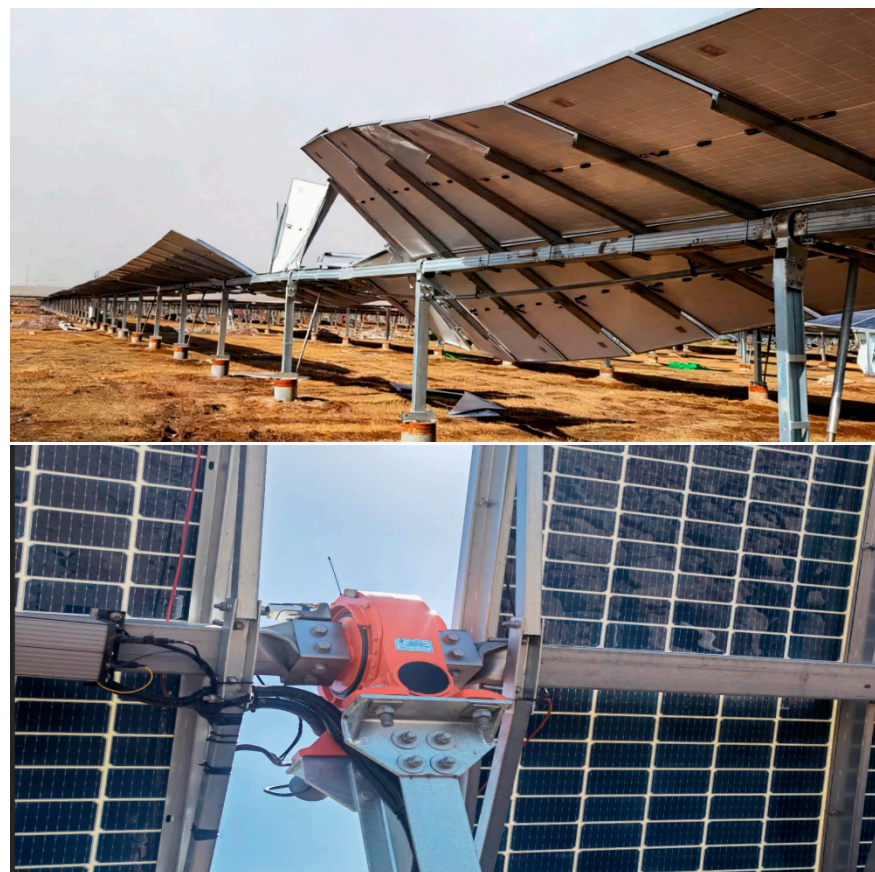
Figure 1. Scene after wind-induced failure.
