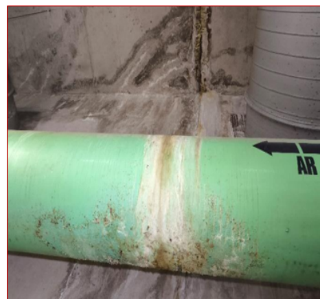
Figure 7. Corrosion case found in the HSP segment.
