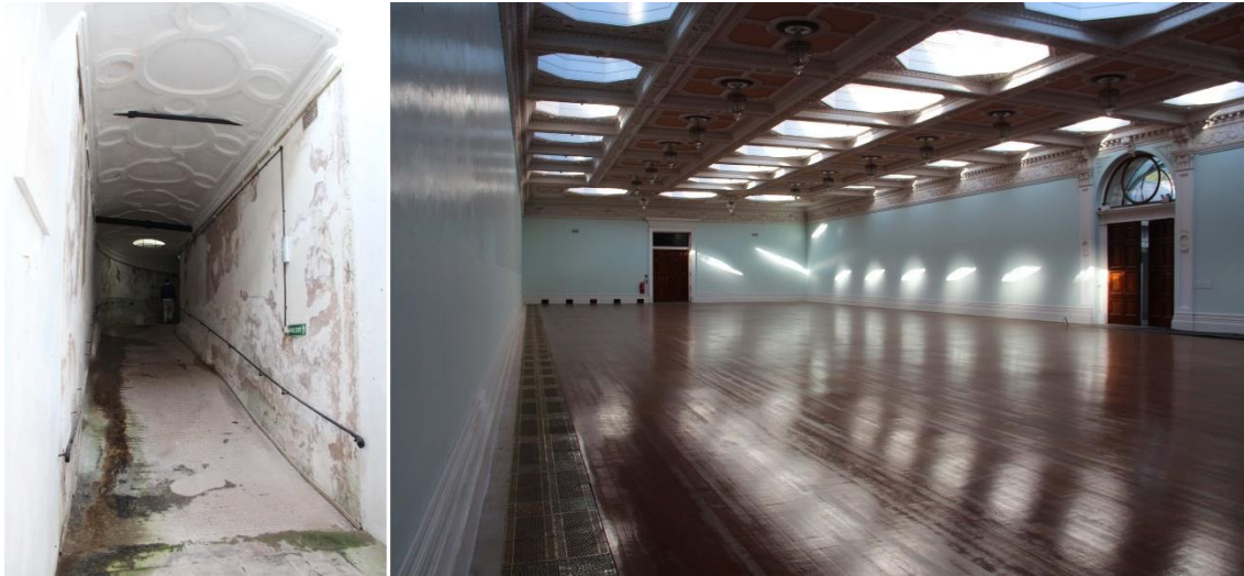
Figure 10. Underground ballroom. The huge room, covering approximately 1200 square meters, was originally intended to fit the new chapel. The ceiling was built with large metal beams. The photographs, taken by the author in October 2015, show its current condition.
