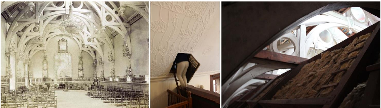
Figure 8. Titchfield Library, 1896. (left) The old Riding Hall was converted into a library and chapel by the 5th Duke of Portland (Manuscripts and Special Collections, University of Nottingham, Nottingham). (center) Hatch into the false ceiling. In the images taken during the author's visit in October 2015, the wooden beams have disappeared. (right) A new roof, carved with natural and divine images, hovers over our heads, molding space with a new shape.
