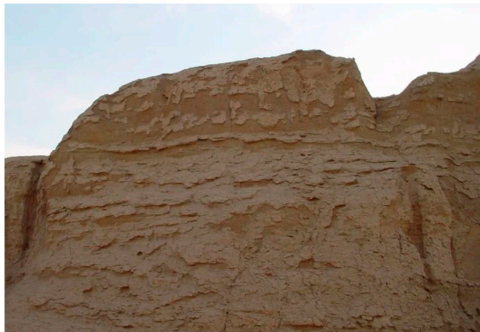
Figure 2. Current spalling conditions at the Yar City site [4].
