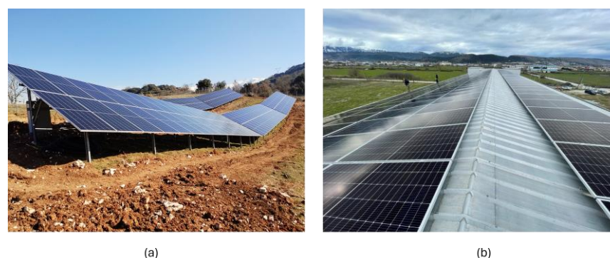
Figure 2. Koutselio ground-based (a) and Mpaфра rooftop (b) PV installations (99.83 kWp and 99.90 kWp, respectively).
