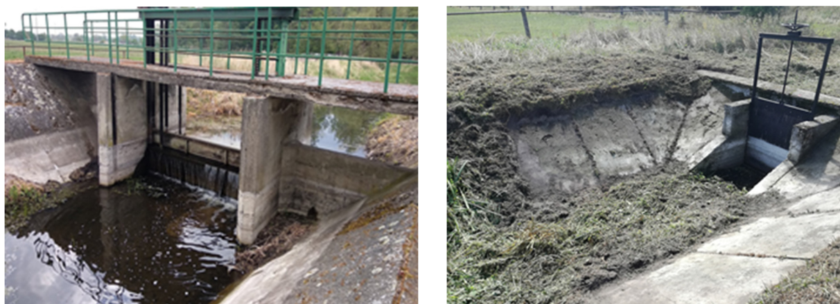
Figure 2. Photos of water structures S4—Weir on the Wyskoć Ditch and S3—water gate on the Racocka Struga River.
