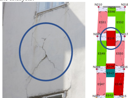
Figure 25. Comparison of the damaged spandrel (Eastern façade).
