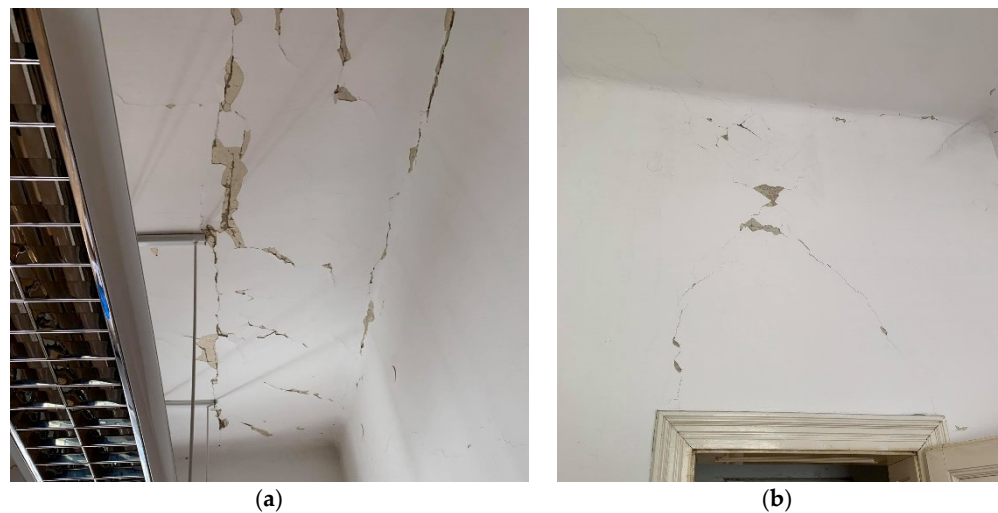
Figure 7. Cracks in the ceiling (a) and above the openings (b) on the 2nd floor.
