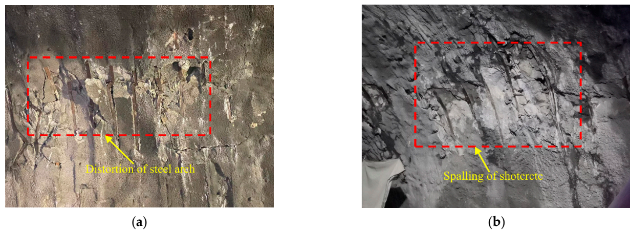
Figure 3. Typical hazard photos of the Yongfeng Tunnel: (a) twisted side wall arches; (b) arch waist sprayed concrete falling blocks.
