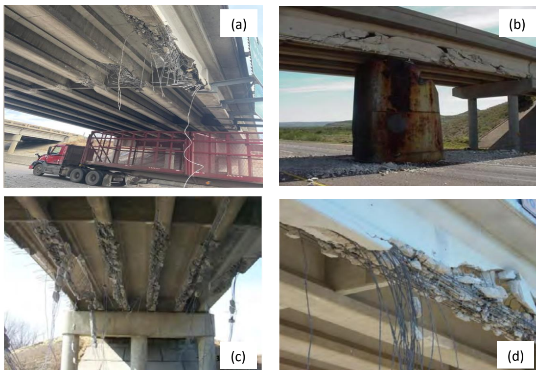
Figure 1. Examples of over-height truck collisions with bridge superstructures [40]: (a) I-10 overpass at I-49, Lafayette; (b) RM215 over IH10, Pecos Co, TX; (c) Sgt. Bluff bridge, IA; and (d) FM479 over Kerr Road, San Antonio, TX.
