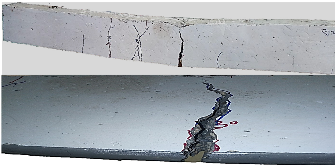
Figure 11. Mode of failure of beam CB2d.
