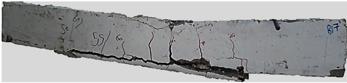
Figure 21. Mode of failure of beam B17.
