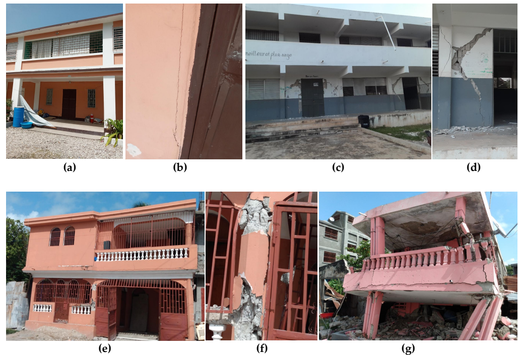
Figure 7. Building damage states: (a,b) minor, (c,d) moderate, (e,f) severe, (g) partial or total collapse [42].
