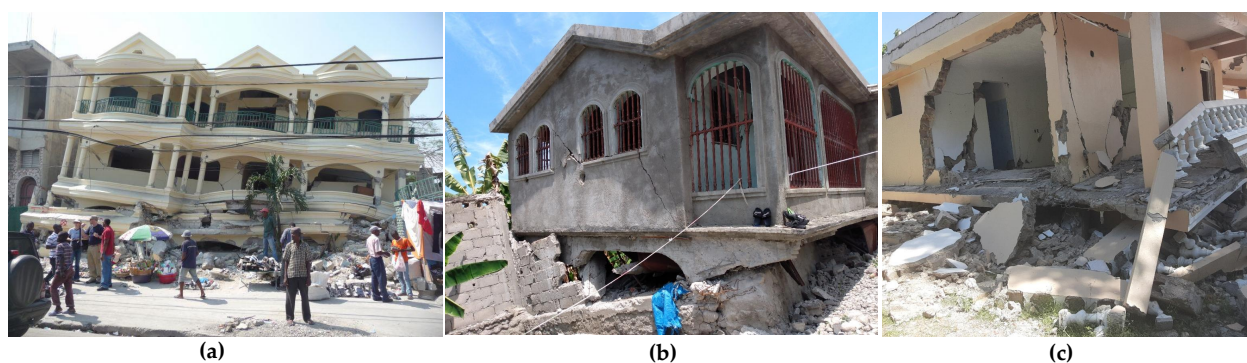
Figure 3. Soft-story failure during the (a) 2010 and (b,c) 2021 earthquakes [1,2].
