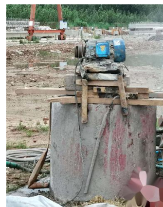
(b) Vertical slurry tank and motor
