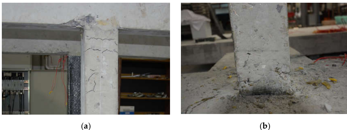
Figure 8. Column damage under the CFRP retrofitted model: (a) damage to the bottom of the beam; (b) column bottom damage.
