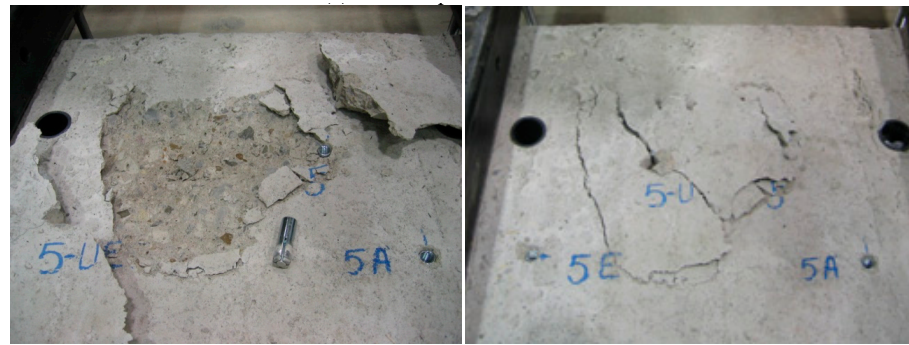
(b) Concrete breakout after the ultimate tension test
