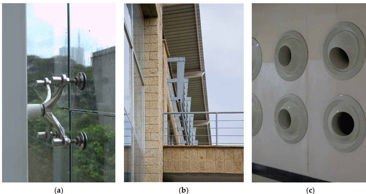
Figure 14. (a) The 12 mm thick glass curtain wall. (b) Aluminium louvers with roof overhang. (c) Evaporative cooling units. Source: Author 2023.
