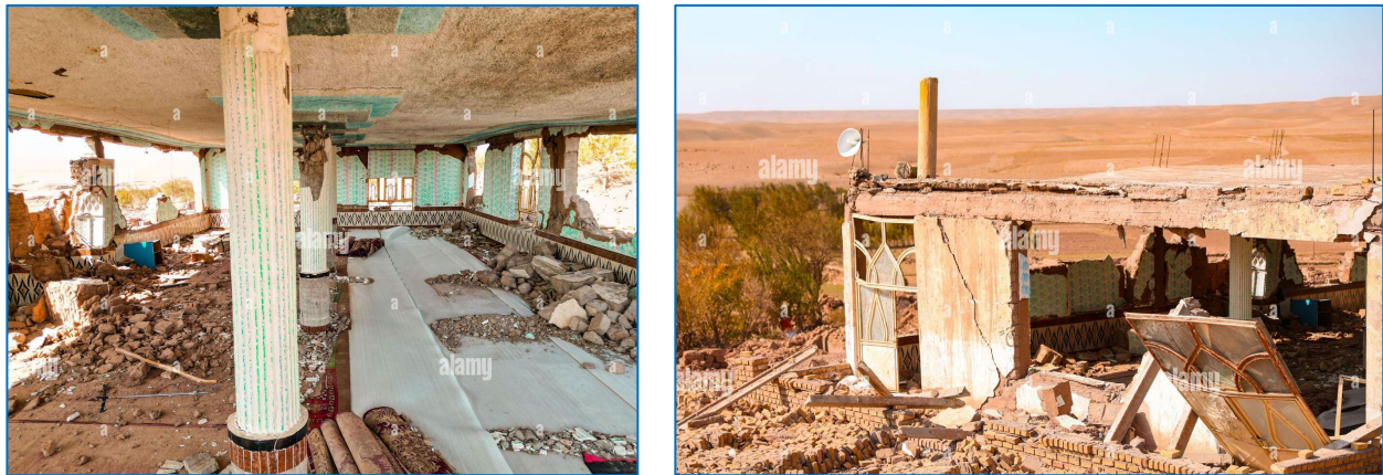
Figure 1. Masonry-infilled RC Masjid building damaged in the Herat Earthquake, 2023 (taken by https://www.alamy.com/ , accessed on 15 September 2024).
