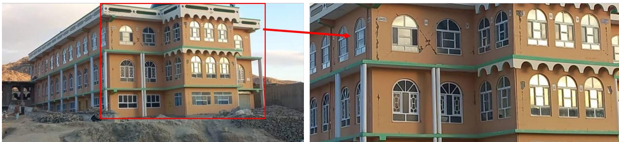
Figure 2. Masonry-infilled RC Gian Masjid building damaged in the Paktia Earthquake, 2022.
