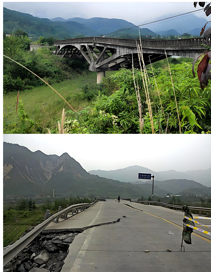
Figure 1. Severely damaged Xiaoyudong Bridge after the 2008 Wenchuan earthquake. (An example of a “critically damaged” state on the verge of collapse).
