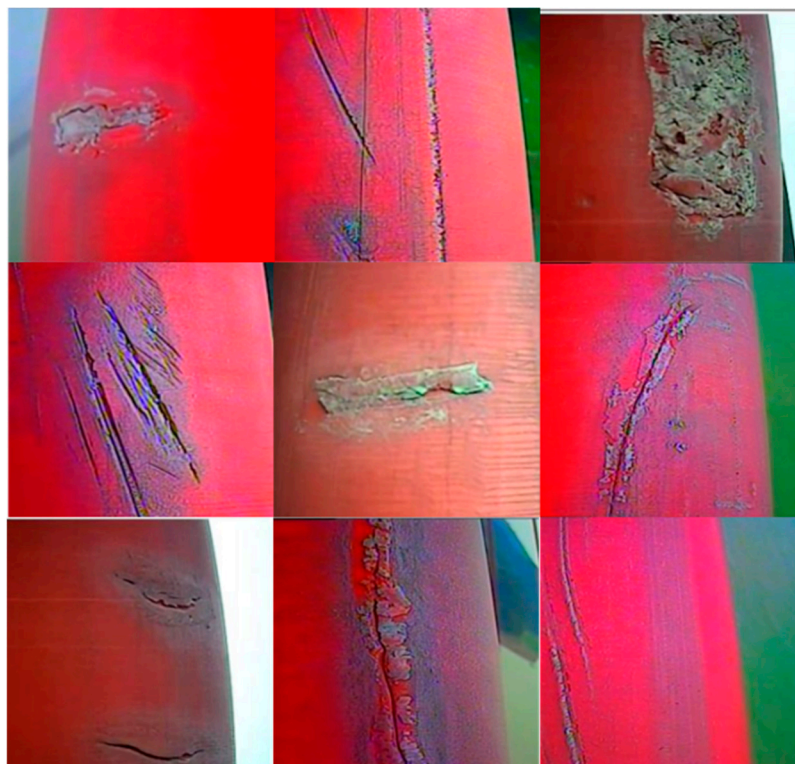
Figure 1. HDPE sheath cracking.
