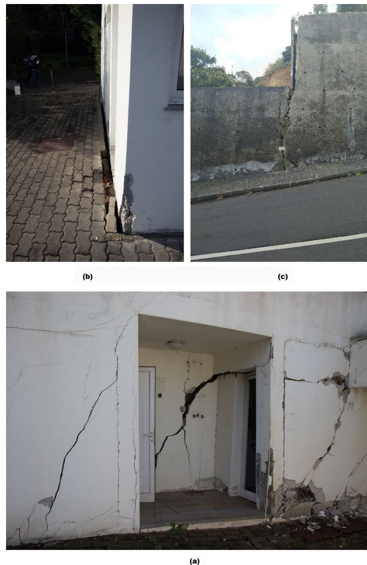
Figure 5. Forensic documentation of structural pathologies (2013–2022): (a) Severe diagonal tension and shear cracks in masonry structures; (b) Ground surface rupture and pavement settlement caused by active deep-seated creep; (c) Structural separation and outward tilting of legacy retaining walls (Source: Photographic survey adapted from CMM technical reports).
