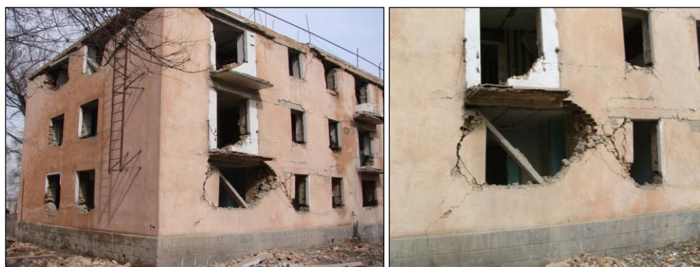
Figure 11. Typical object damage.
