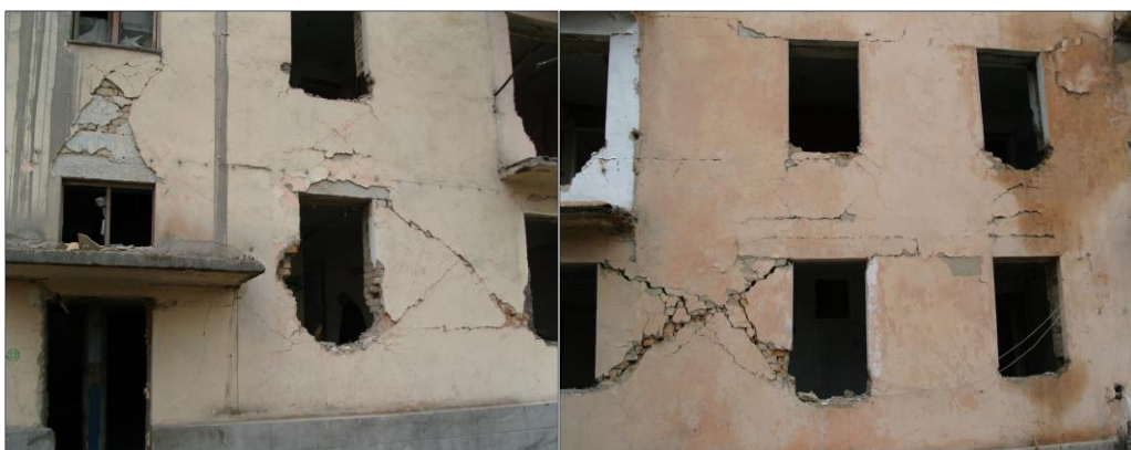
Figure 10. Typical object damage (diagonal cracks).
