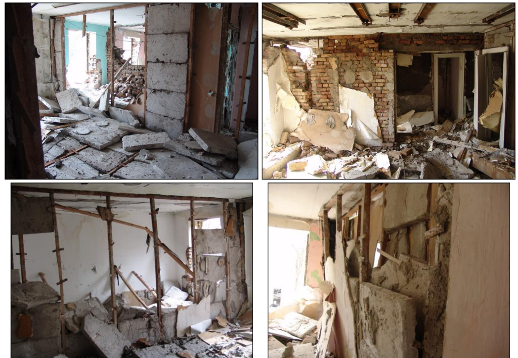
Figure 12. Damage inside the building.
